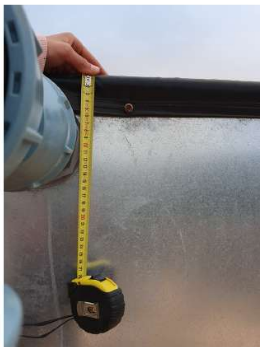
Picture 31 Dam 1 Overflow 15 cm from top
