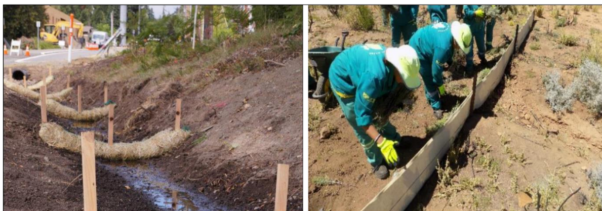
Figure 23. Examples of silt socks (left) and a silt fence (right) placed perpendicular to the flow of water. These methods reduce the force of water flow, erosion and can prevent unwanted sedimentation a site.
