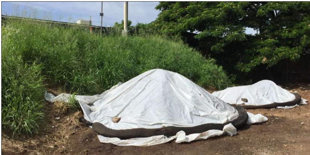
Figure 22. Stockpiles of fine textured building materials and soils covered with geotextile/plastic covering and bunded with sandbags when not in use.
