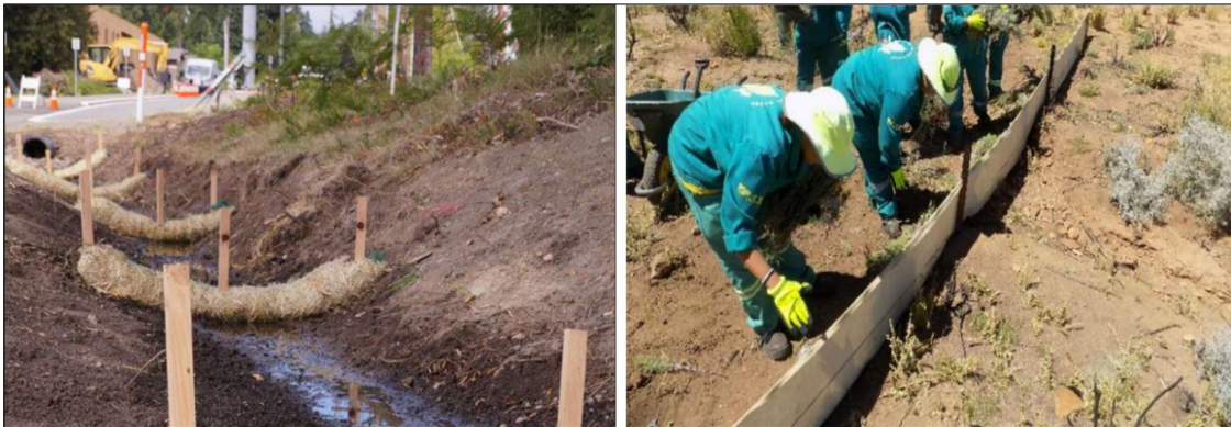
Figure 21. Examples of silt socks (left) and a silt fence (right) placed perpendicular to the flow of water. These methods reduce the force of water flow, erosion and can prevent unwanted sedimentation a site.
