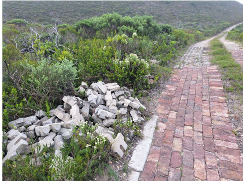
Figure 24. Inappropriate disposal or storage of pavers used during road maintenance activities.
