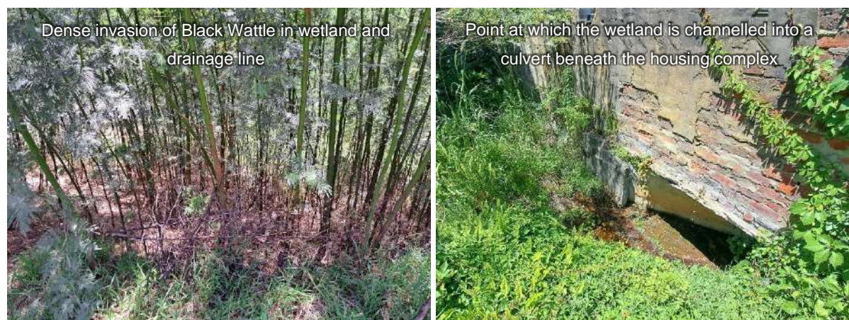
Figure 19. Photos of the wetland and drainage lines indicating impacts affecting the Present Ecological State of the wetland.
