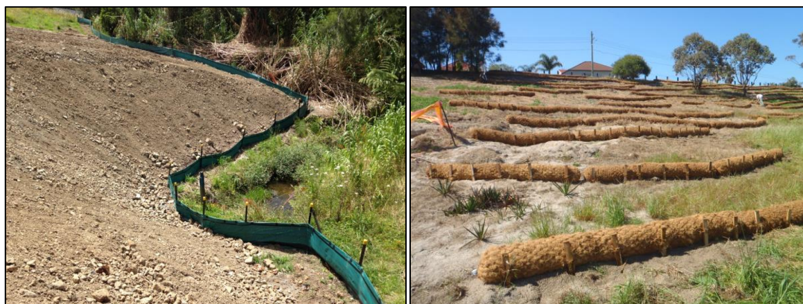
Figure 24: Examples of silt fences (left) and coir logs (right) used to trap sediment mobilised from steep slopes.
