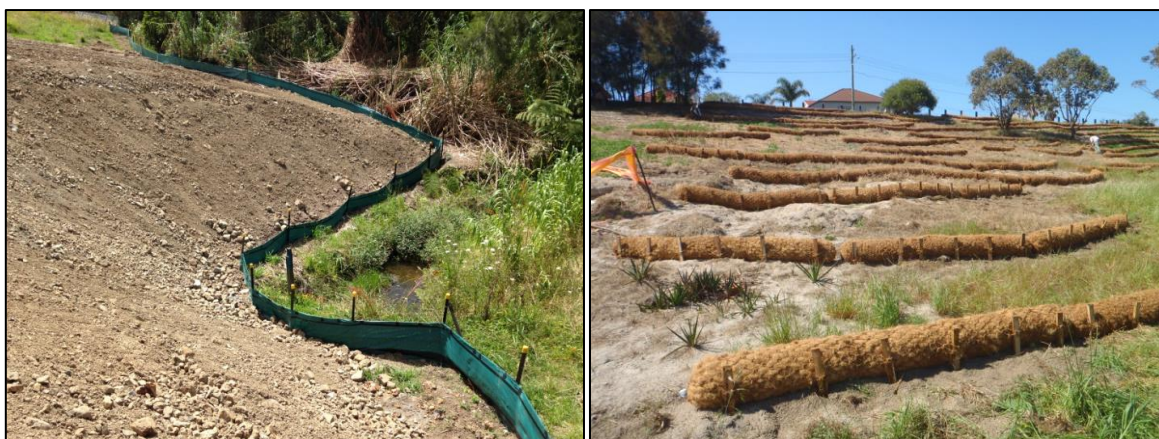
Figure 18: Examples of silt fences (left) and coir logs (right) used to trap sediment mobilised from steep slopes.
