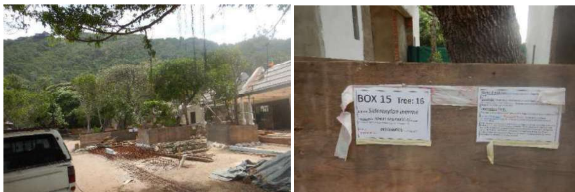
Figure 14: Images of a construction site where protected and indigenous trees were marked and protected on the site.
