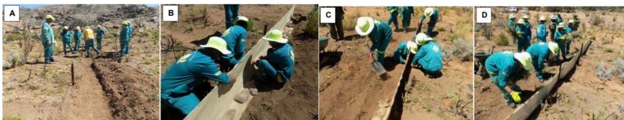
Figure 12: Installation of the soil erosion control fence. A: Installing the standards and wires and preparing the trench. B: Fitting the geotextile, tying it on with wire. C: Filling in the trench over the geotextile. D: Applying a mulch against the completed fence (Photos courtesy Ken Coetzee).
