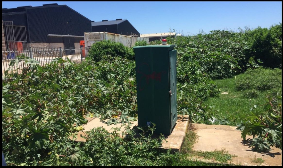
Figure 4: Tarragona Sewer Pump Station
