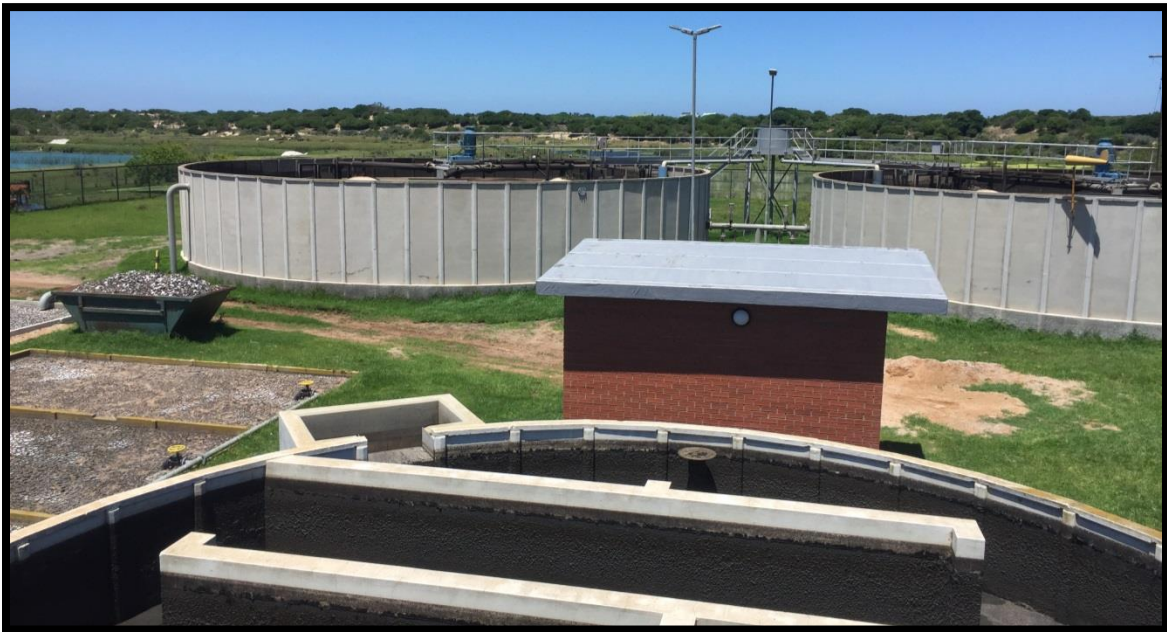
Figure 3: St Francis WWTW
