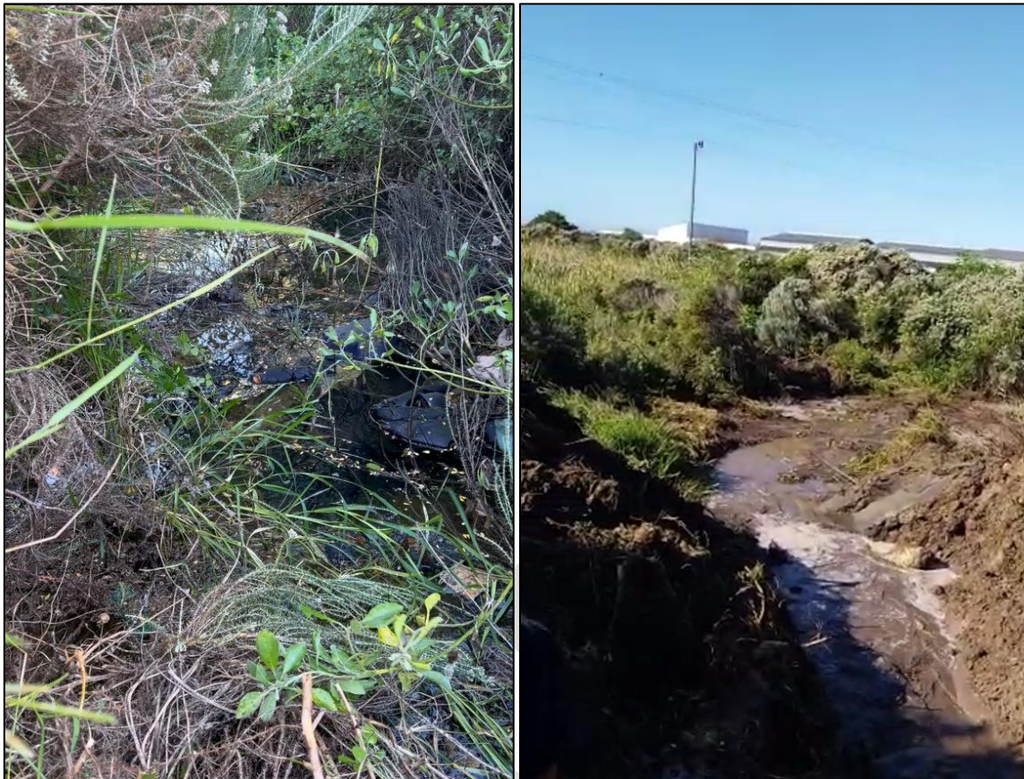
Figure 7: Stills from video footage obtained of the leak to the west of Wetland A. The T. capensis reed-beds from Wetland A can be observed in the background of the right image.
