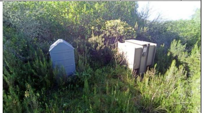
17. Electrical boxes / "housing" on the eastern boundary of Erf 1058 (Dr. Peter Nilssen).
