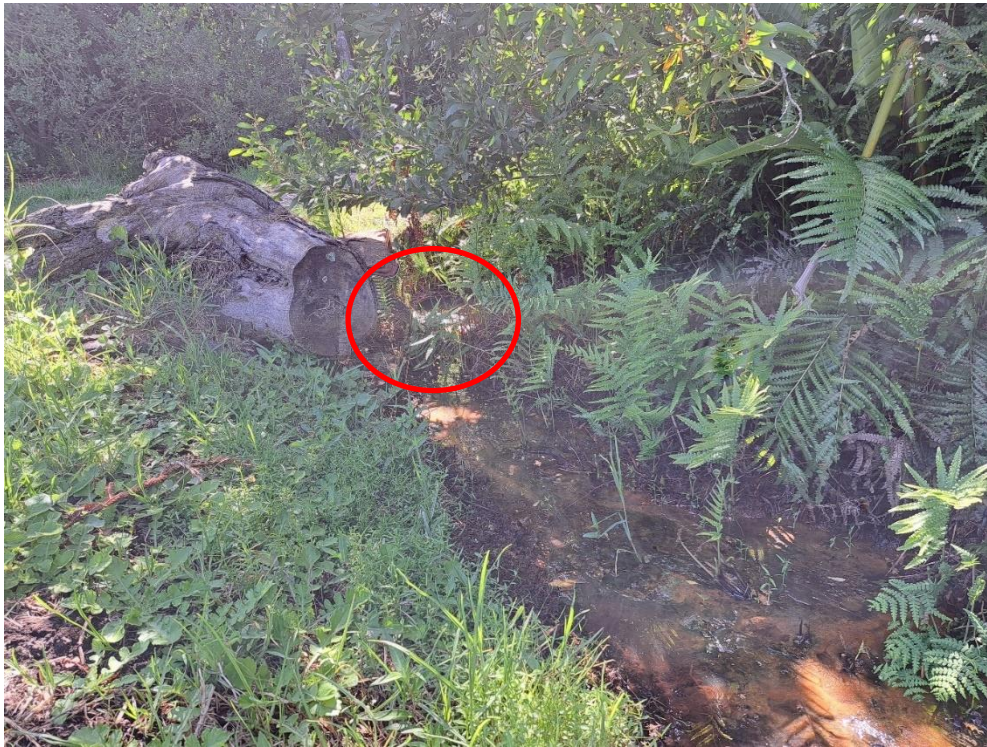
Figure 11: Photograph of the western-most culvert blocked by vegetation and sediment.
