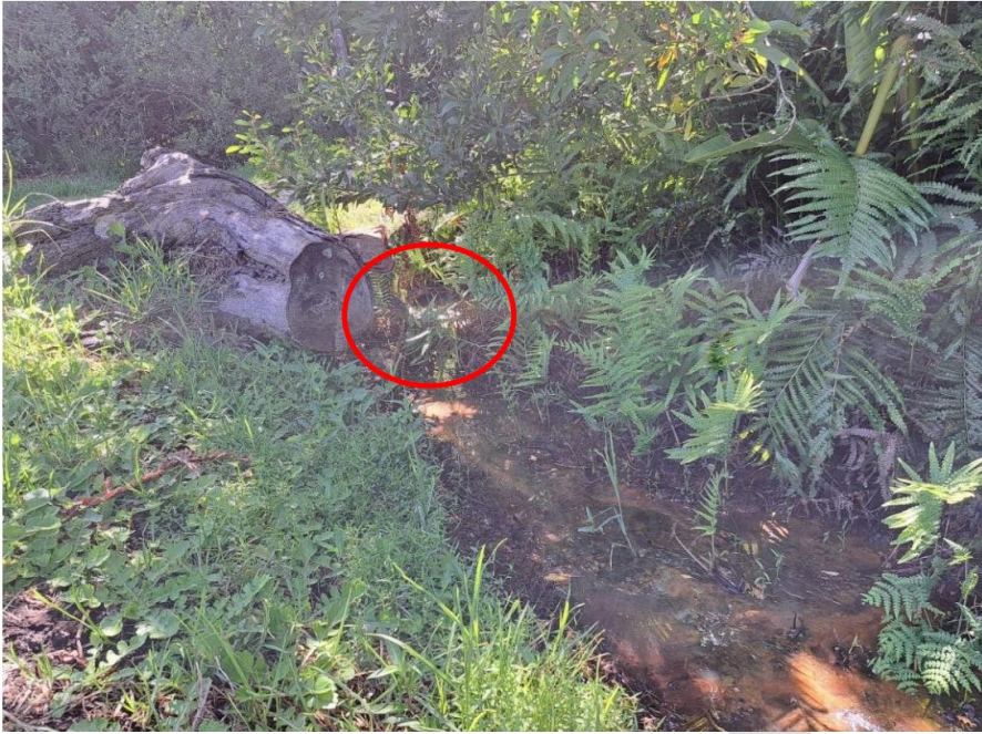
Figure 13: Photograph of the western-most culvert blocked by vegetation and sediment.
