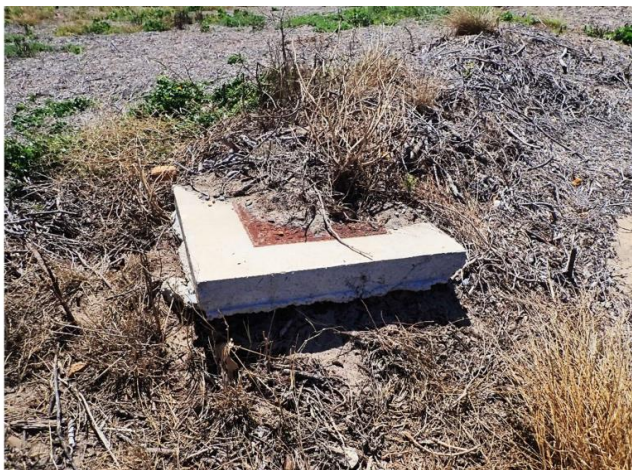
Figure 7: Bulk service installed on site prior to March 2006.
