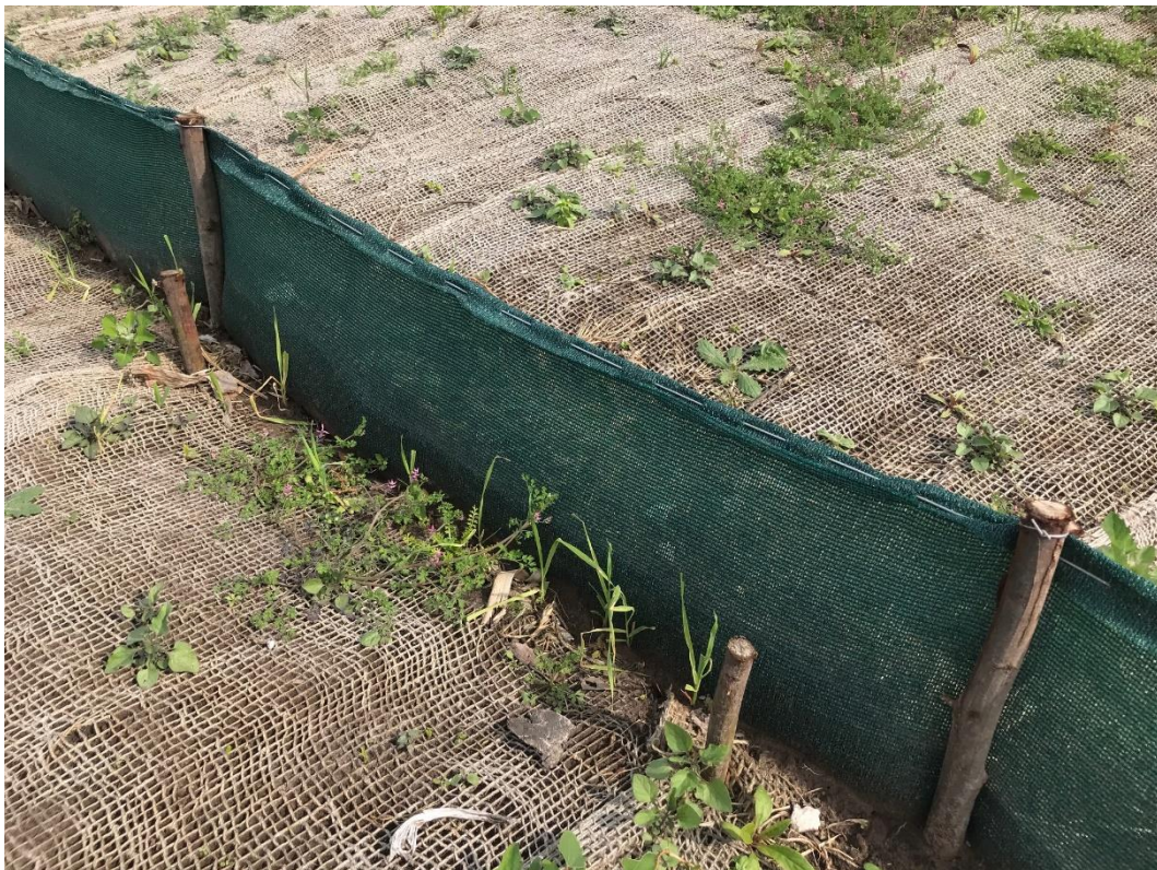
Figure 17. Images of installed soil saver matting and silt fences several weeks after installation.
