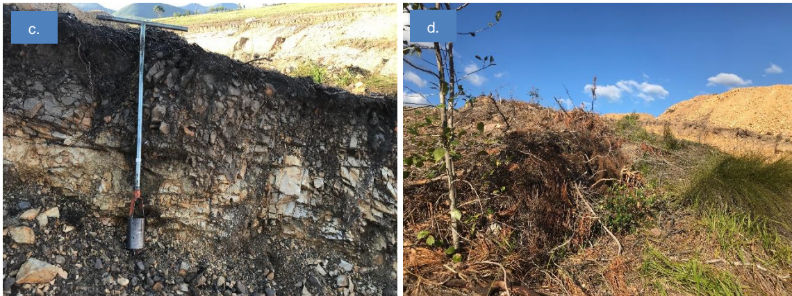
Figure 13. Photos of the site indicating a: the extent of earthworks across the valley effectively eliminating the watercourse channel and bed; b: the lower portion of the excavated area showing the natural vegetation beyond; c: the depth of strip excavations in relation to a soil auger (130 cm), and d: a small area of remnant vegetation on topsoil with some dead pine trees interspersed with indigenous trees and grasses.
