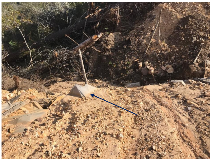
Figure 11. Overwhelmed silt curtain at the outflow of the dam excavation.
