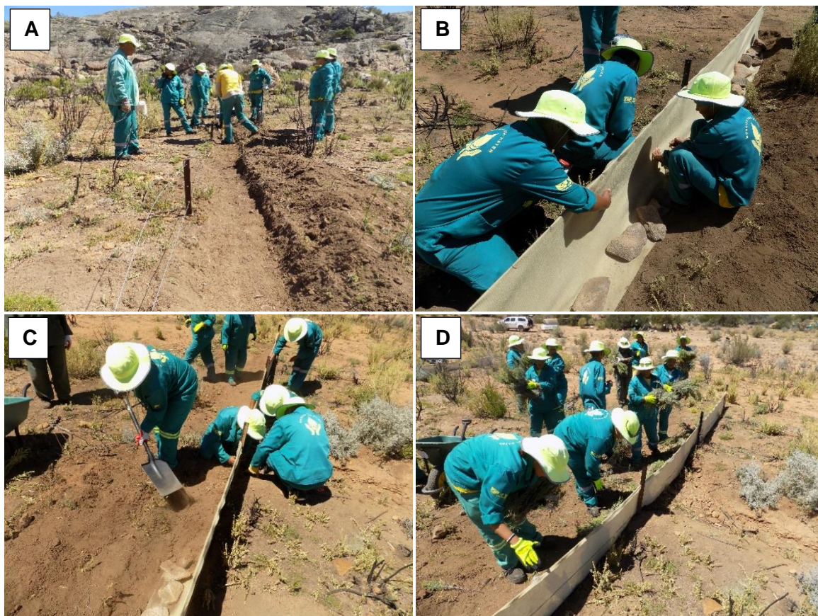
Figure 19. Installation of the soil erosion control fence. A: Installing the standards and wires and preparing the trench. B: Fitting the geotextile, tying it on with wire. C: Filling in the trench over the geotextile. D: Applying a mulch against the completed fence (Photos courtesy Ken Coetzee).
