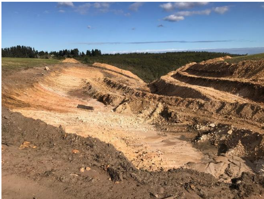
Figure 2. Photo taken of the excavated dam basin showing disturbance of topsoil, subsoil and rock, and the removal of vegetation (17 June 2021).
