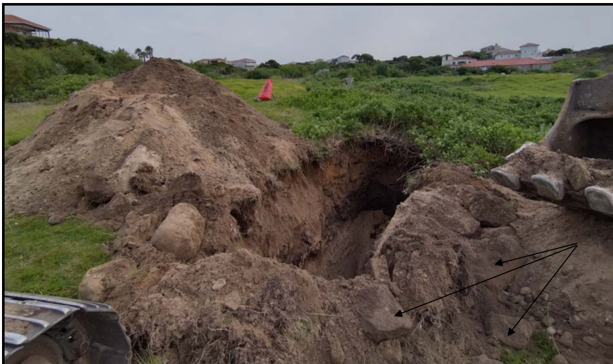
Figure 11: Boulders and calcrete/calcarene rock encountered at the base of some pits
