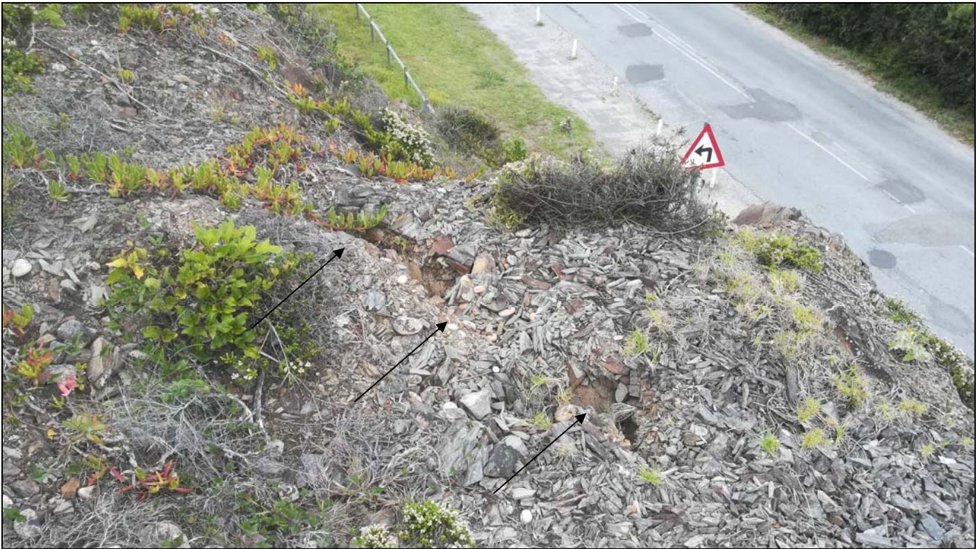
Figure 8: Tension crack along the edge of very steep slope on southern boundary
